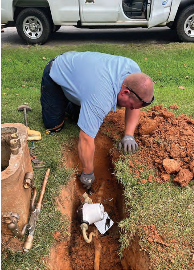
Before updating the service connection, a Meter Technician exposes the water meter and service lines.
